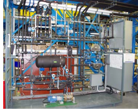
Fig. 2. Overall view of experimental set-up.
